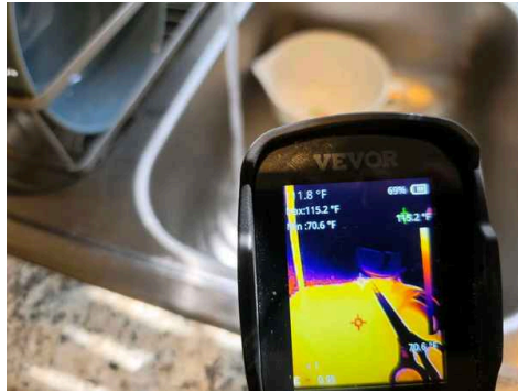
Water Heater Functioned
