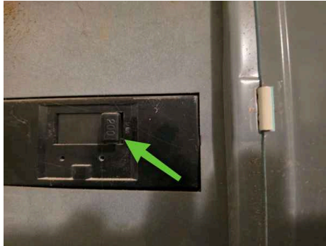
Main Power Shut-off
