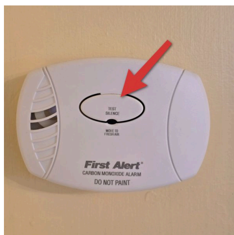
Failed to respond to the TEST BUTTON
