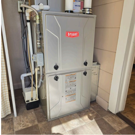
The Furnace was visually inspected, but NOT TESTED. Gas OFF at the time of the inspection
