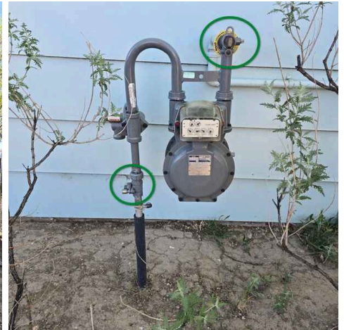
Main Gas Valve
