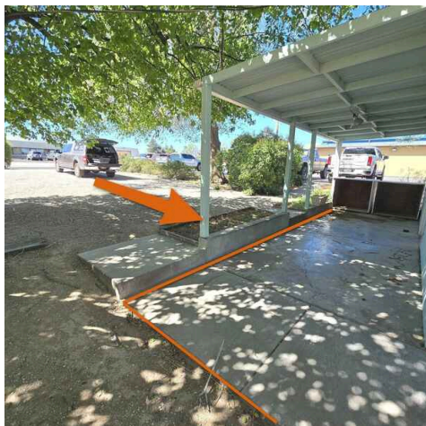
Direction of slope: Elevation drop at front of house from driveway.
