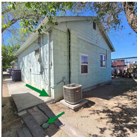
An underground drain system has been installed for the rain gutters on the east side, which leads to a pop-up drain on the downhill (north) side of the house.
