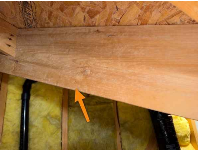
5.10.1/7.4.1 - Mold-like growth. This is old on dry wood, and the cause was rectified when the roof was re-done and is documented in pictures by Patriot Roofing. The surface was wiped clean with bleach.
