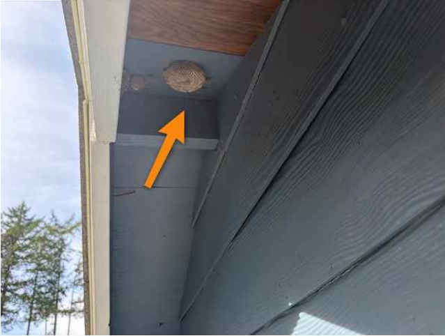
4.26.1 – Pests. Two wasp/hornet nests were removed when the roof was cleaned.
