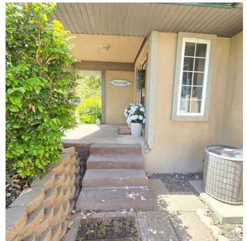
4 Risers Present, a handrail is recommended
