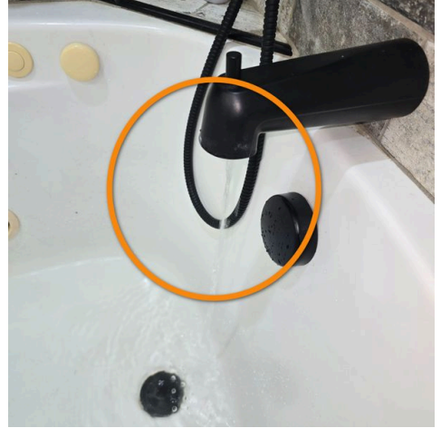
Water Flow almost completely stops before well kicks in
