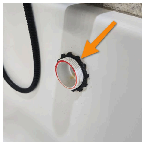
Compression Nut Cracked: Overflow Seal Jeopardized
