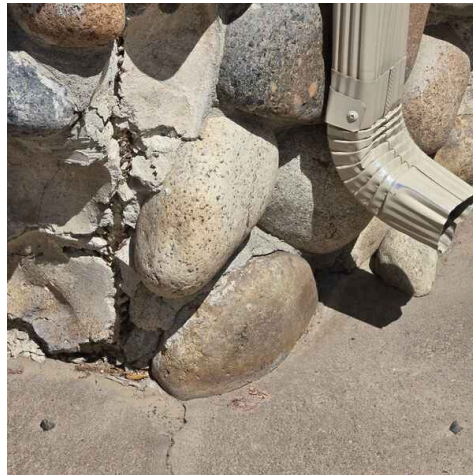
A Closer Look: Cracking and stone delamination
