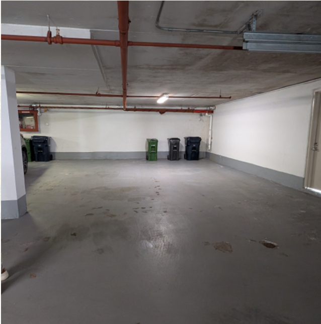
2 Underground Side by Side Parking Spots Length 22'3 Ft X Width 18'6 Ft (Approx)
