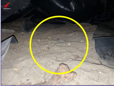
The vapor barrier is missing or damaged on the crawlspace floor. The vapor barrier is used to prevent ground moisture from moving up and into the living area of the home. Recommend a licensed contractor install a proper vapor barrier.
