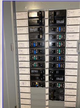
Main panel view.
