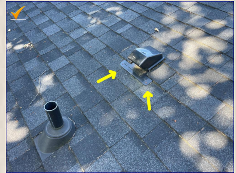
There are exposed nail heads securing the flashing to the roof. Exposed nail heads can allow water to penetrate the roof. Recommend a licensed roofer repair as necessary.
