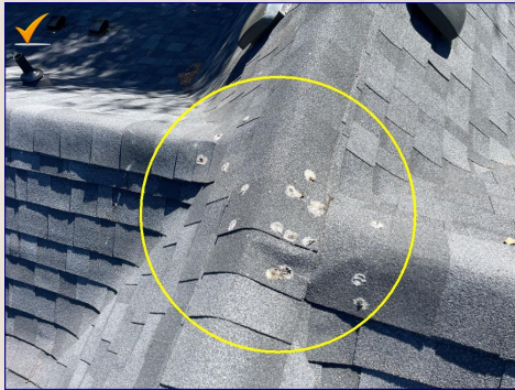
There are exposed nail heads on the roof. Exposed nail heads may allow water to seep through and damage the sheathing over time. Recommend a licensed roofer evaluate and repair as needed.
