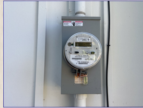
The electrical service entrance
