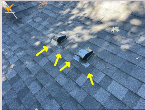
There are exposed nail heads securing the flashing to the roof. Exposed nail heads can allow water to penetrate the roof. Recommend a licensed roofer repair as necessary.
