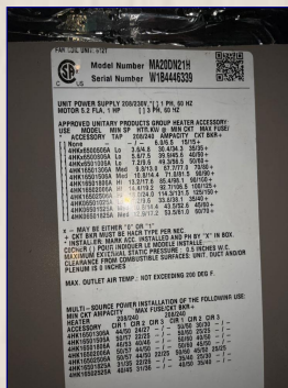
The furnace, data tag
