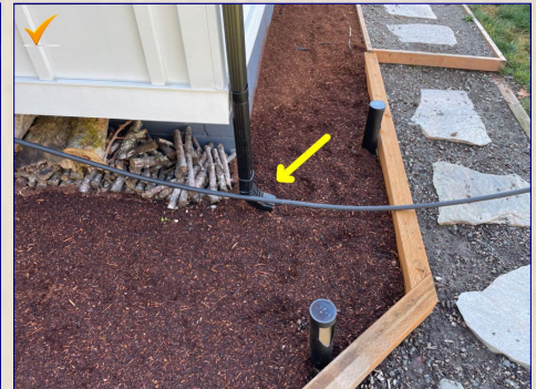
The gutter downspouts don't direct water far enough away from the house. Recommend adding downspout extensions (5-6' extensions recommended) to discharge away from the home.
