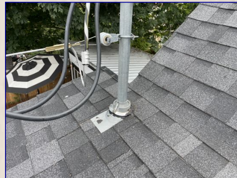
The service entrance boot had been repaired.
