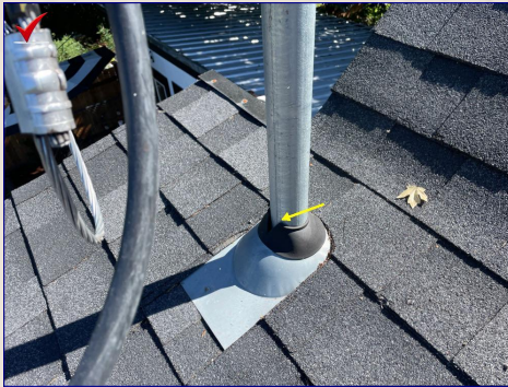
There are one or more areas of the roof flashing in need of sealing/repairs. Risk of water damage. Recommend a licensed roofer evaluate and repair or replace the flashing as needed.
