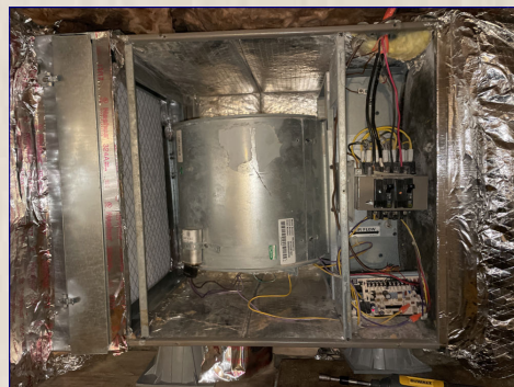
The furnace view, cover off
