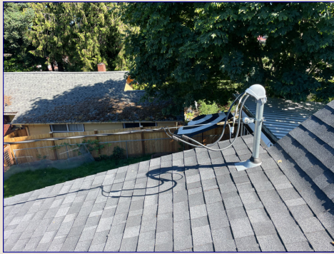
The electrical service entrance
