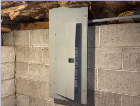
Main panel view.
