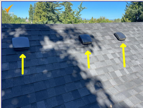
There are exposed nail heads securing the flashing to the roof. Exposed nail heads can allow water to penetrate the roof. Recommend a licensed roofer repair as necessary.
