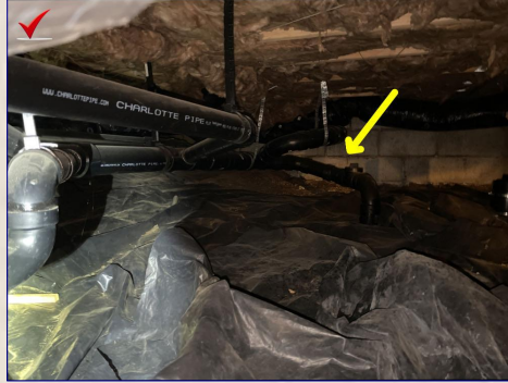
The vapor barrier is missing or damaged on the crawlspace floor. The vapor barrier is used to prevent ground moisture from moving up and into the living area of the home. Recommend a licensed contractor install a proper vapor barrier.
