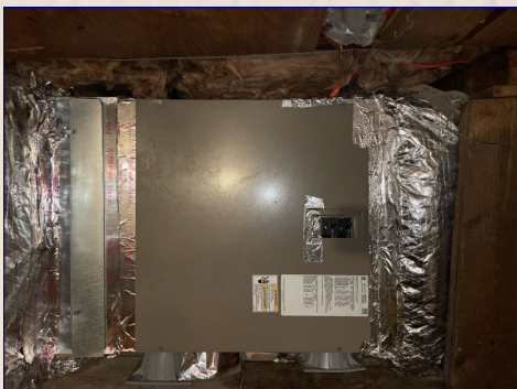
The furnace area
