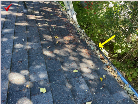
The gutters are dirty. Recommend cleaning the gutters to ensure proper water flow to the downspouts.
