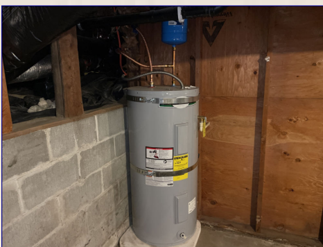
The Water Heater Area
